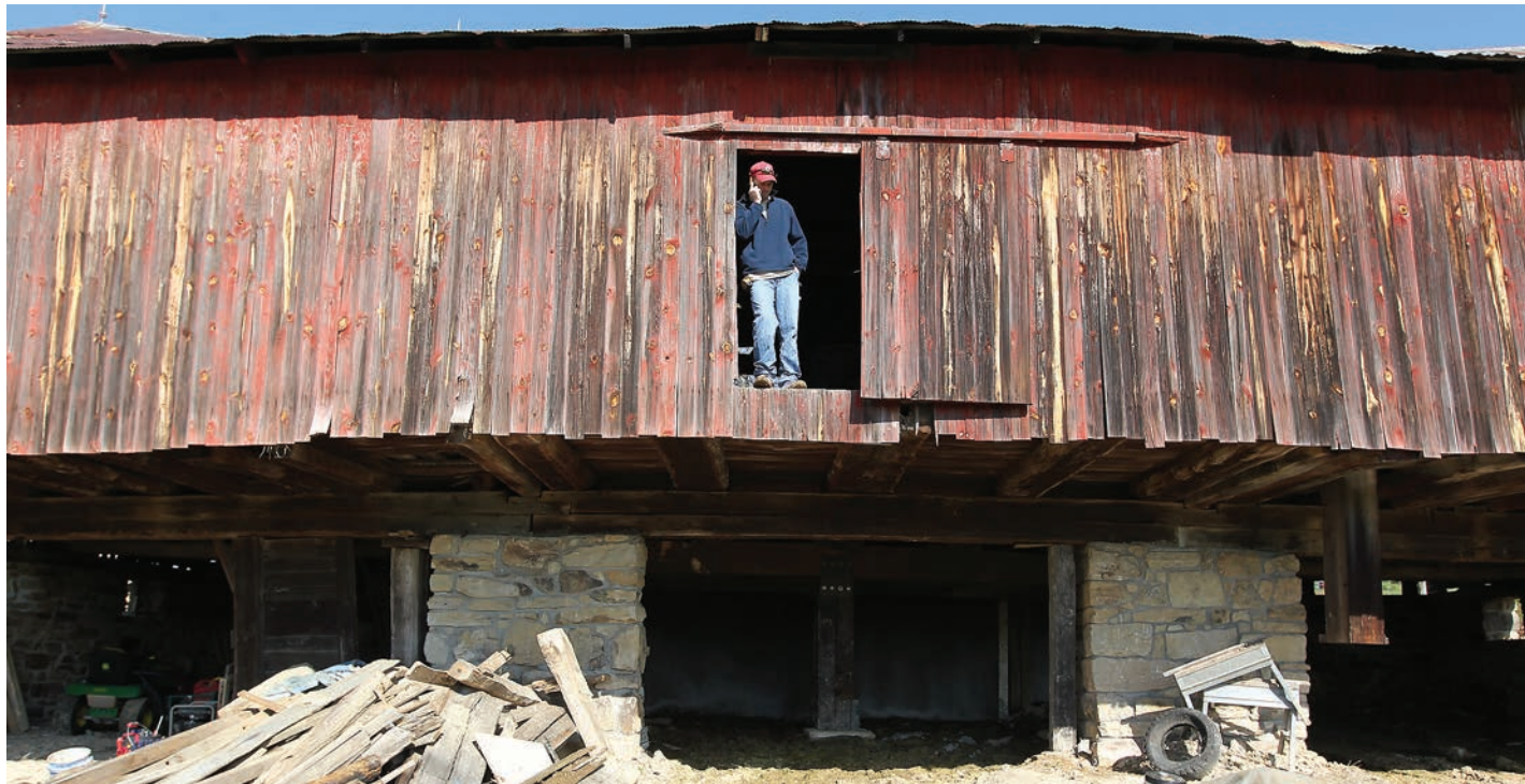
During a restoration project in Ohio, foreman Steve White stands in the hayloft of a barn built in the 1790s near Somerset in Perry County.
